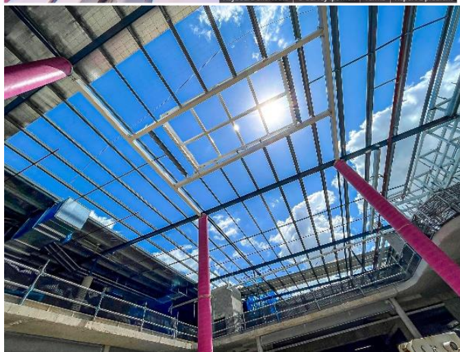
From the roof supports you can see the distinctive shape of the skylight
